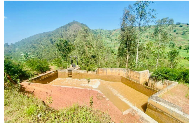
Gaseke HPP generated 1,262,685 kWh in 2022
